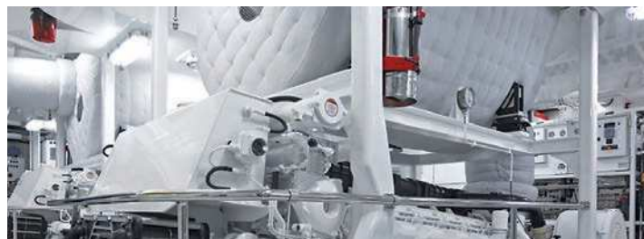
Potential sources of HazMats: cooling systems onboard ships.
